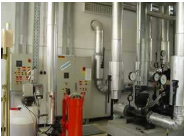
Punct termic modernizat
